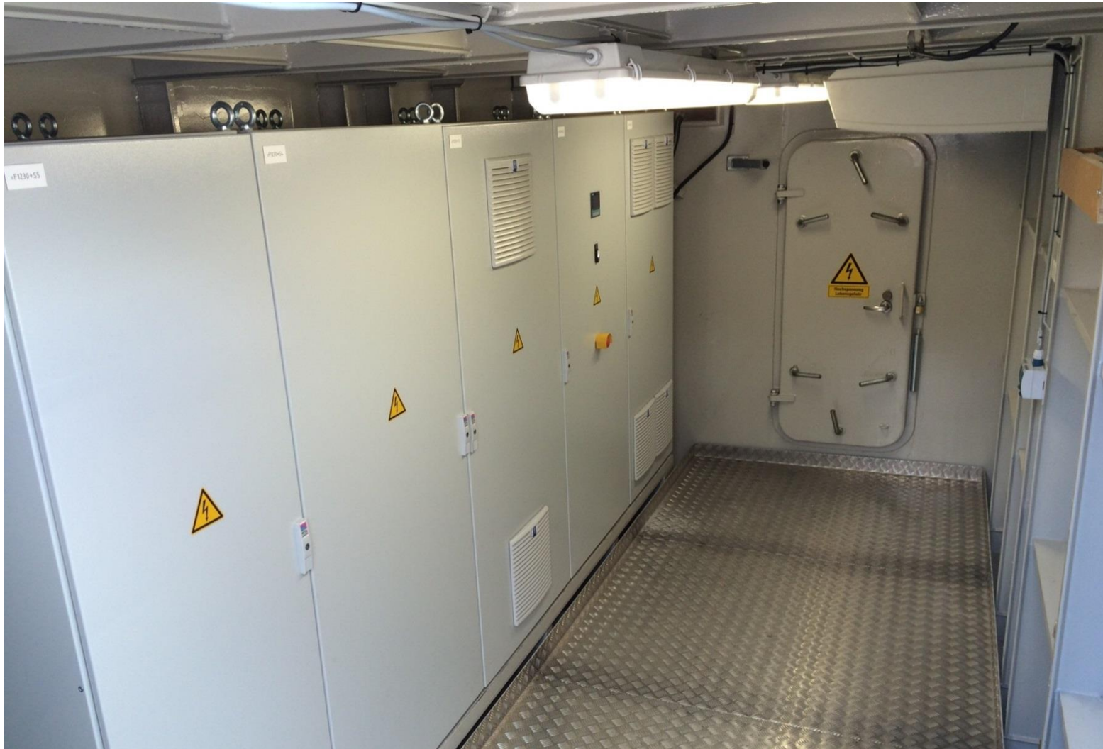
Picture 15-2: Electric pontoon (port) - enclosed design
