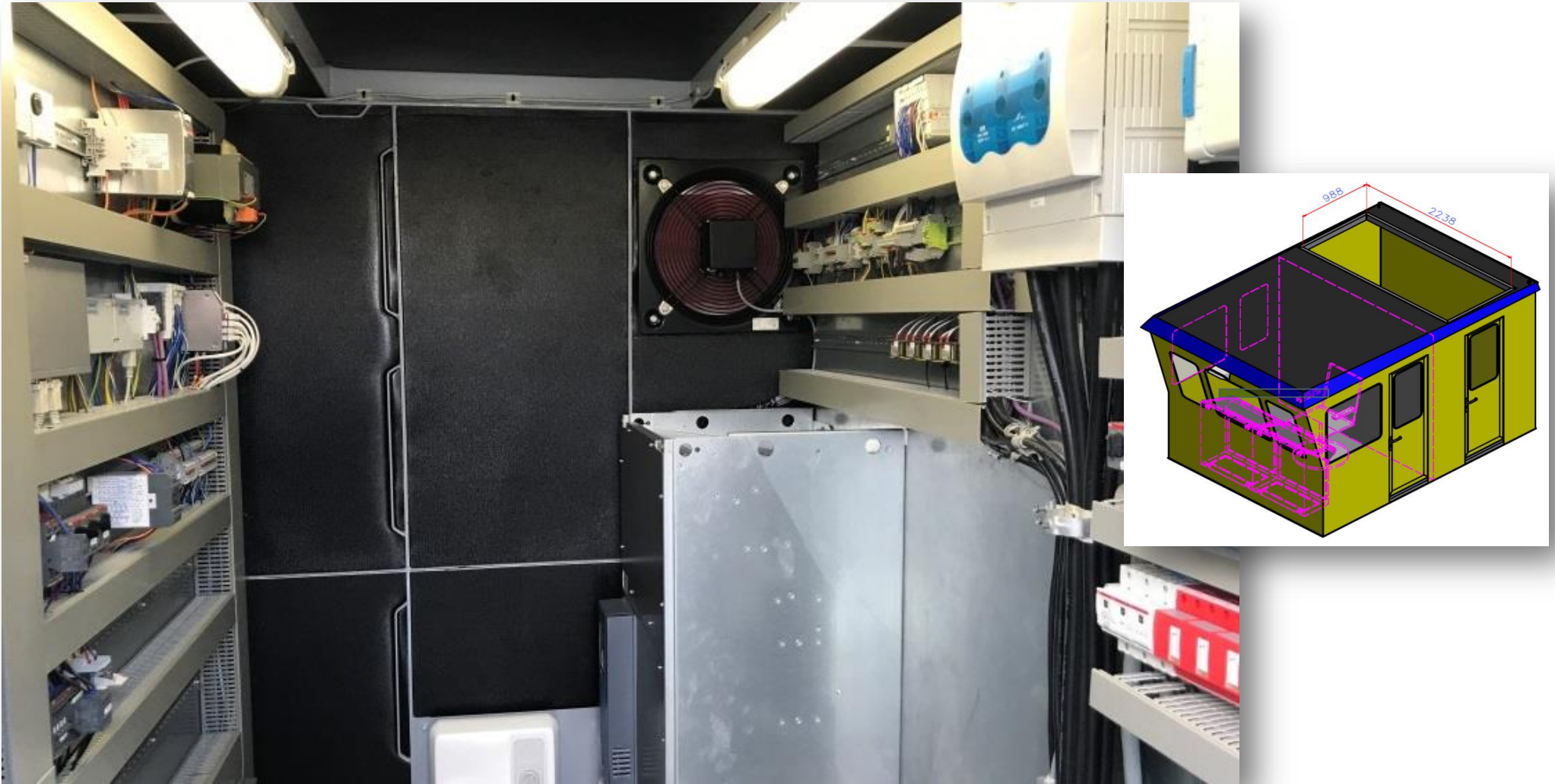
Picture 15-5: Electrical room integrated into the control cabin - open design
