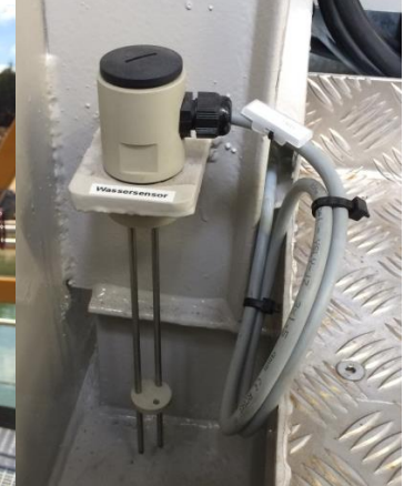
water detector in pontoon
